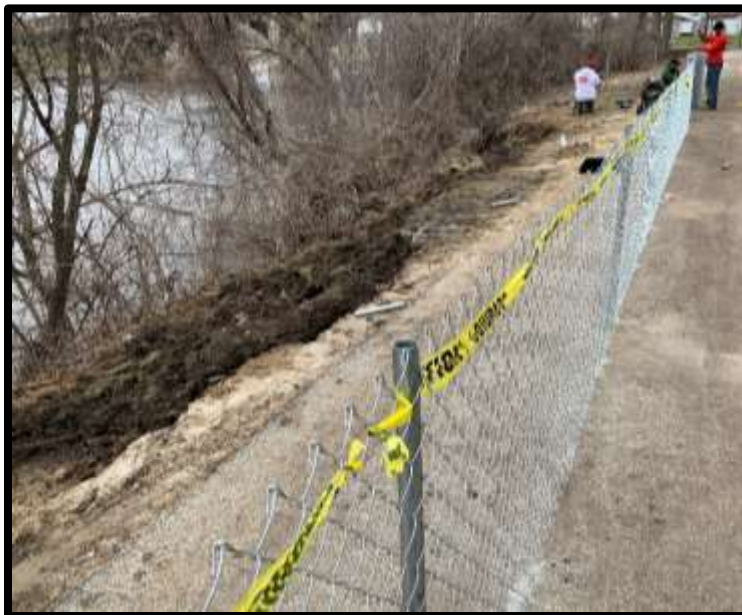
Photo Above: Repair Site
