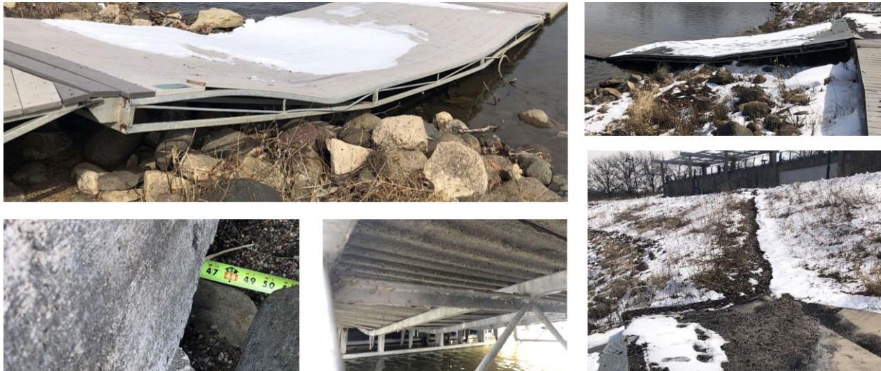
Series of Photos Showing Damage from 2021-2022 Winter Season
