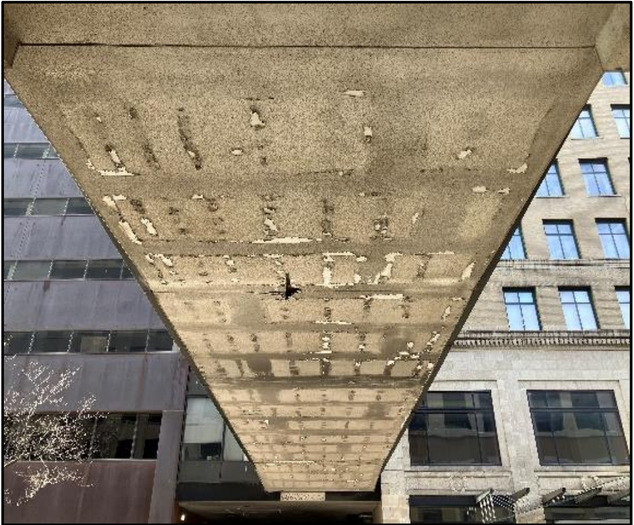
Skywalk Bridge 5E-6E over 6th Avenue (soffit replacement needed)
