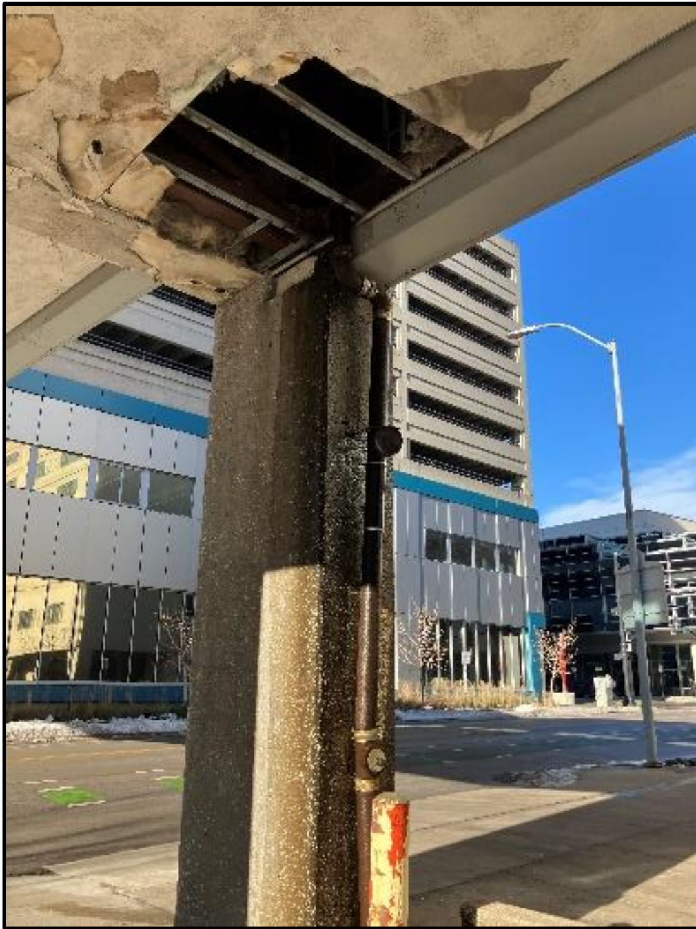
Skywalk Bridge 4E-5E over 5th Avenue (Add-Alternate) (soffit replacement and drainpipe repair needed)
