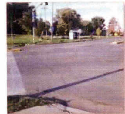
Figure 16. No sidewalk infrastructure
