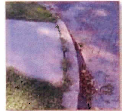
Figure 15. No curb cut
