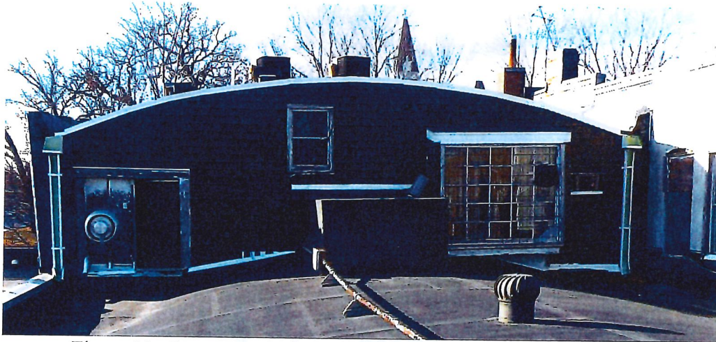
Figure 20: Current upper level east fenestration, looking northwest, building north chimney visible right of center (Jacobsen, 2020)
