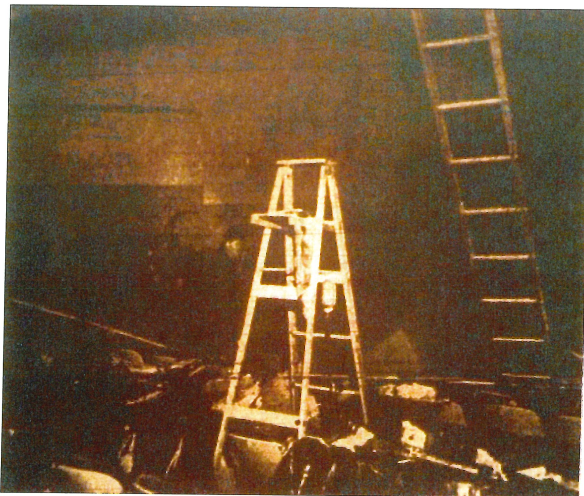
Figure 92: Fire damage in the east auditorium, looking northeast (Des Moines Register, January 23, 1958)
