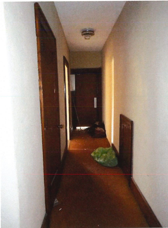
Photo 45: Description: Third floor hall, hall to south stair bay, note infilled door at right, looking south
