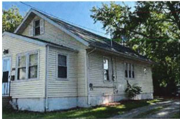
Figure 18. A "before" photo of an ION project to repair a foundation and roof. (Source: City of Des Moines)
