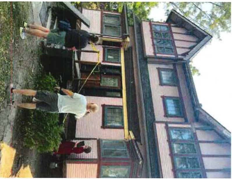
Figure 13. Site meeting with two HPC members and a contractor to discuss an in-progress project in the River Bend neighborhood. (Source: Stacey Hanley)
