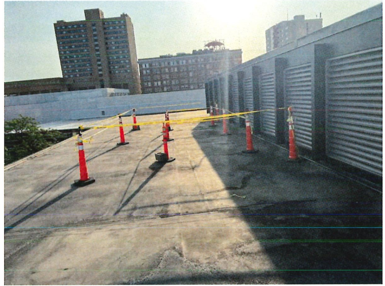
Equipment with screen
